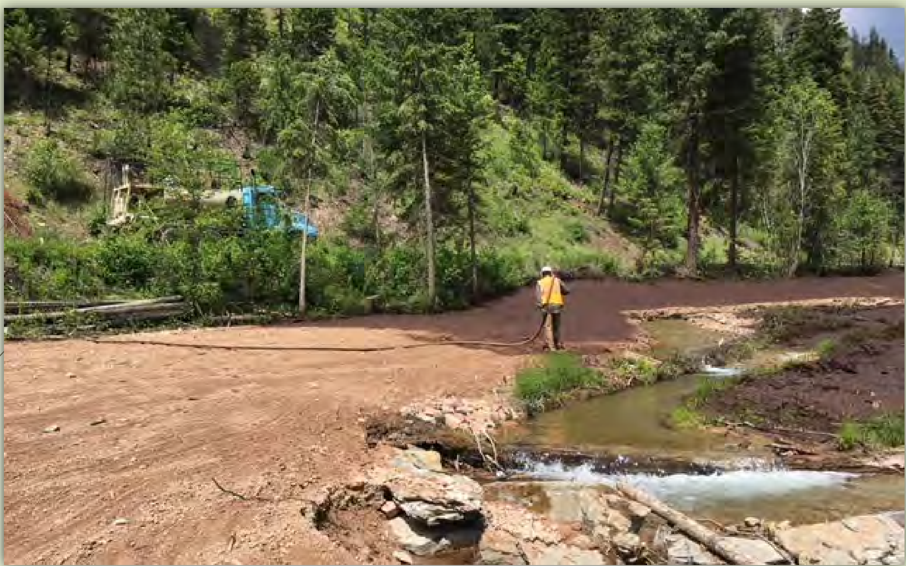
Flat Creek OU2 Project – Contaminated soils removed where possible and remaining contamination capped with imported soils
