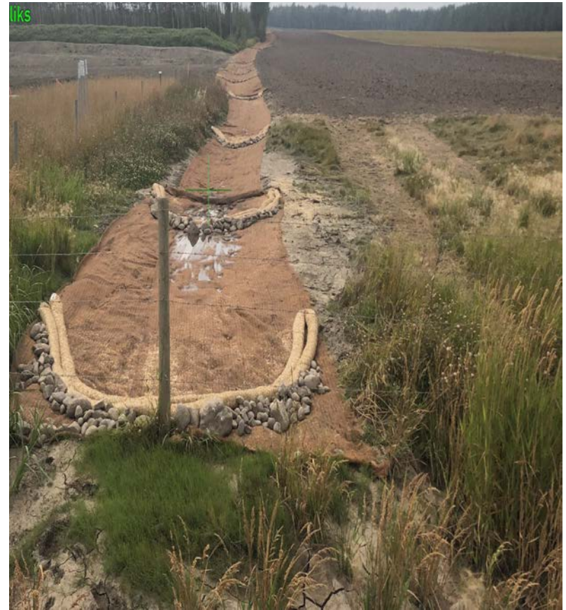
Wattles and low-rise measures - break energy of concentrated flows and allow excess to flow over
