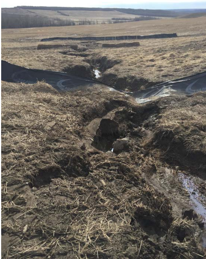
Silt fences/bales - not suitable to break energy of concentrated flows
